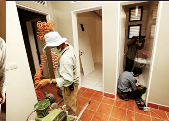
Men at work: staff apply the final touches to Kampot’s newest hospital
